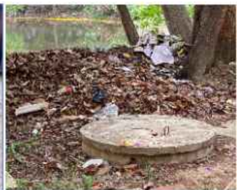
Soak chamber outside Science building for collecting waste
