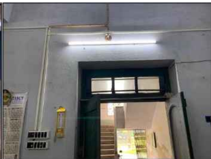
Use of LED at Classroom
