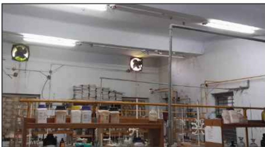
LED light at Chemistry Laboratory
