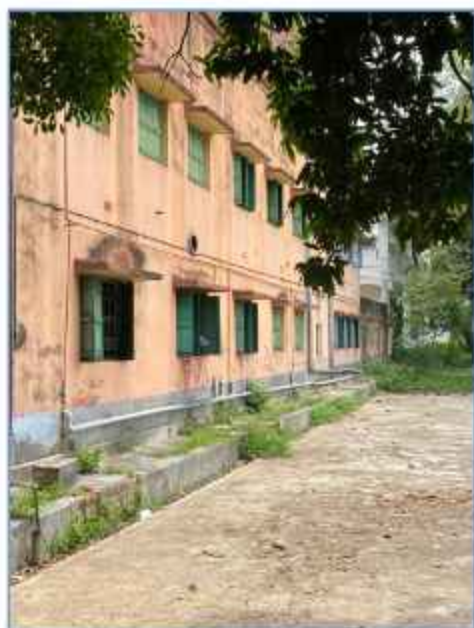
Pipeline outside Ram Mohan building for toilets and canteen
