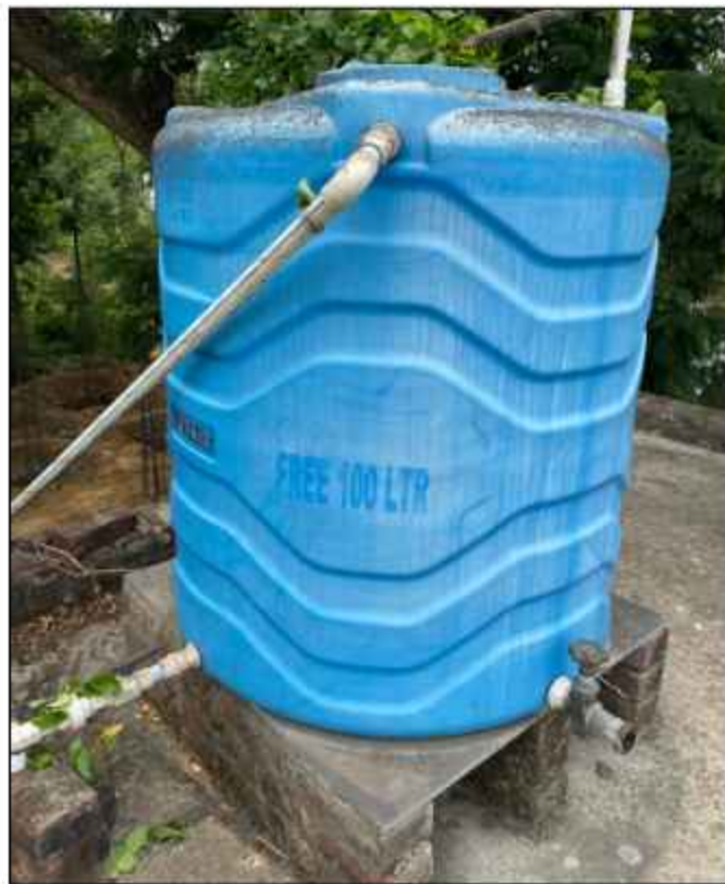
Tank on the roof of Bio-Science Building
