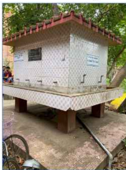
Drinking water reservoir and connected pipeline
